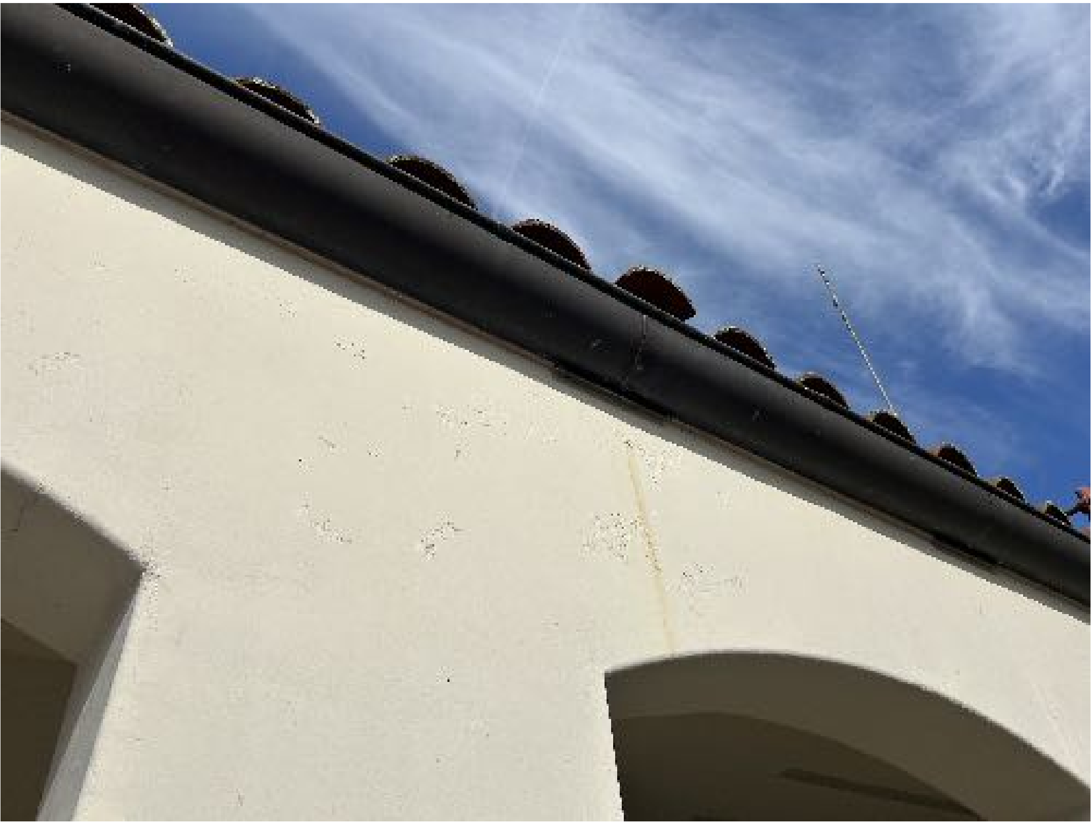
EXISTING GUTTER TO BE RE-SEALED AT CONNECTION
